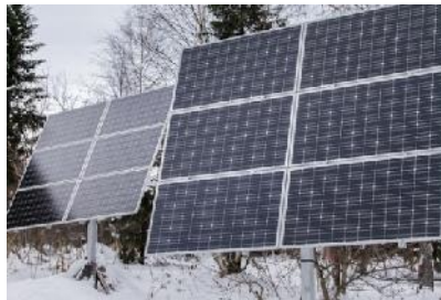
Low temperature effects on PV panels can lead to charge controller damage if the controller is not sized properly.
