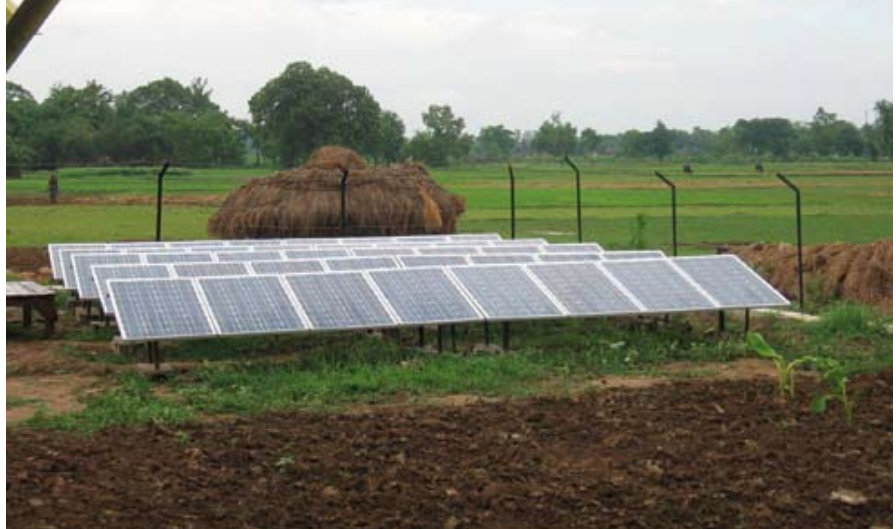
In remote locations, solar energy is the power source of choice. Due to difficult roads, fuel logistics for diesel generators can be a real challenge.
